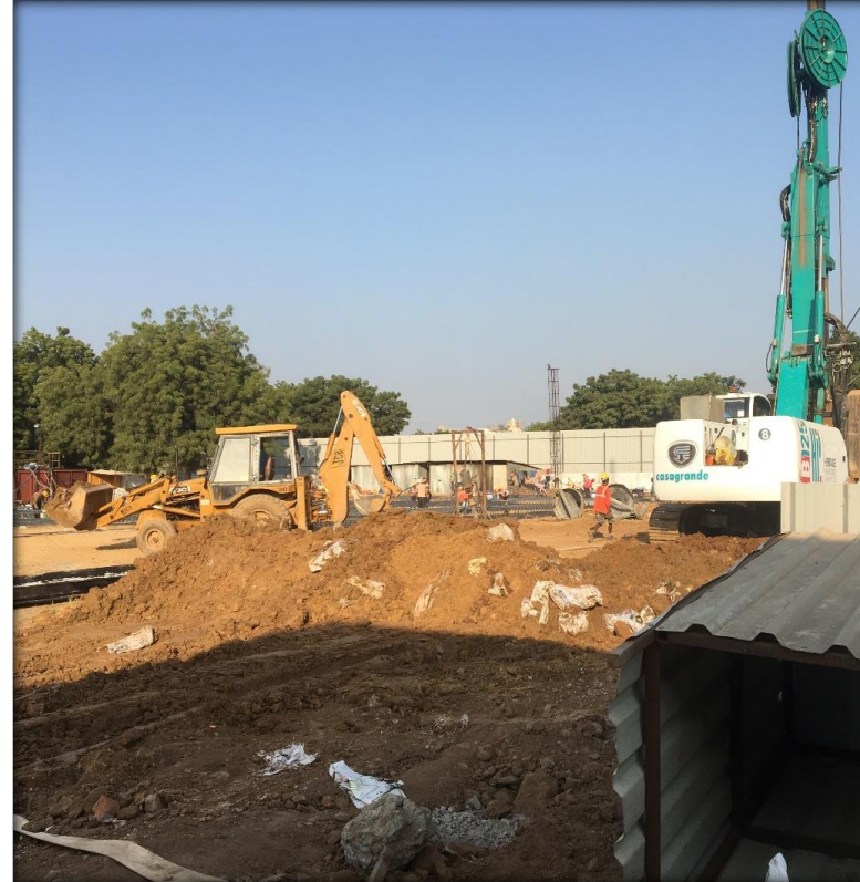
Earth work, Soil excavation, Mobile plant e.g.. Bulldozer, crane, crushers for site clearance work
